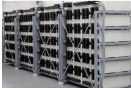
Energy Storage System
